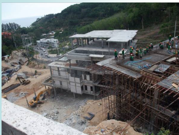
Building A3 in the background – completed Superstructure Building A2 in the foreground – commencing Superstructure
